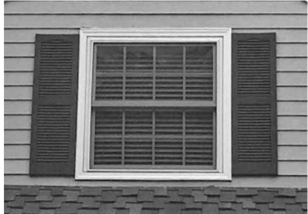
Window with incorrect sized shutters
